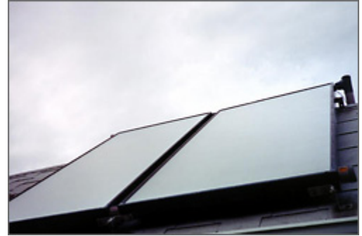
For solar hot water systems, flat-plate solar collectors are typically installed facing south on a rooftop.
